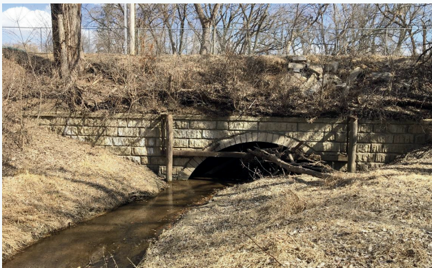
Failing arch culvert in Nebraska City
